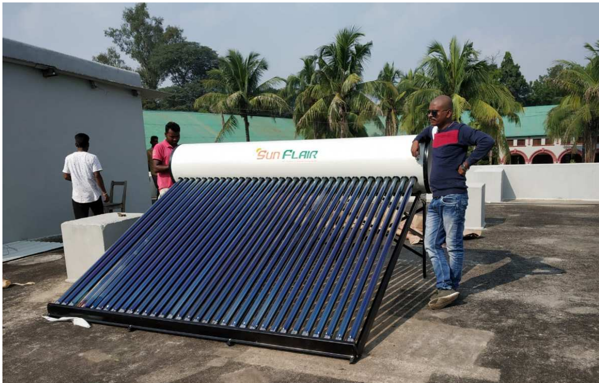
(Solar Water Heater System 500LPD)
